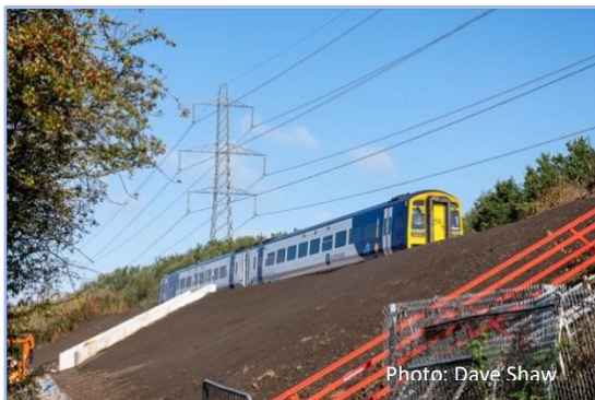
Photo: Dave Shaw A class 158 on a recent tour on the line crosses over a new underpass on the line between Backworth and Seghill.
